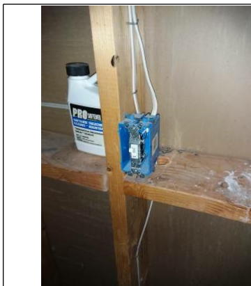
Cover plate missing
