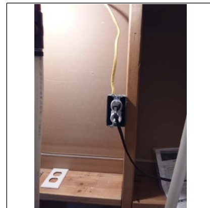
Outlet plate missing
