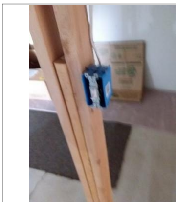
Missing plate cover
